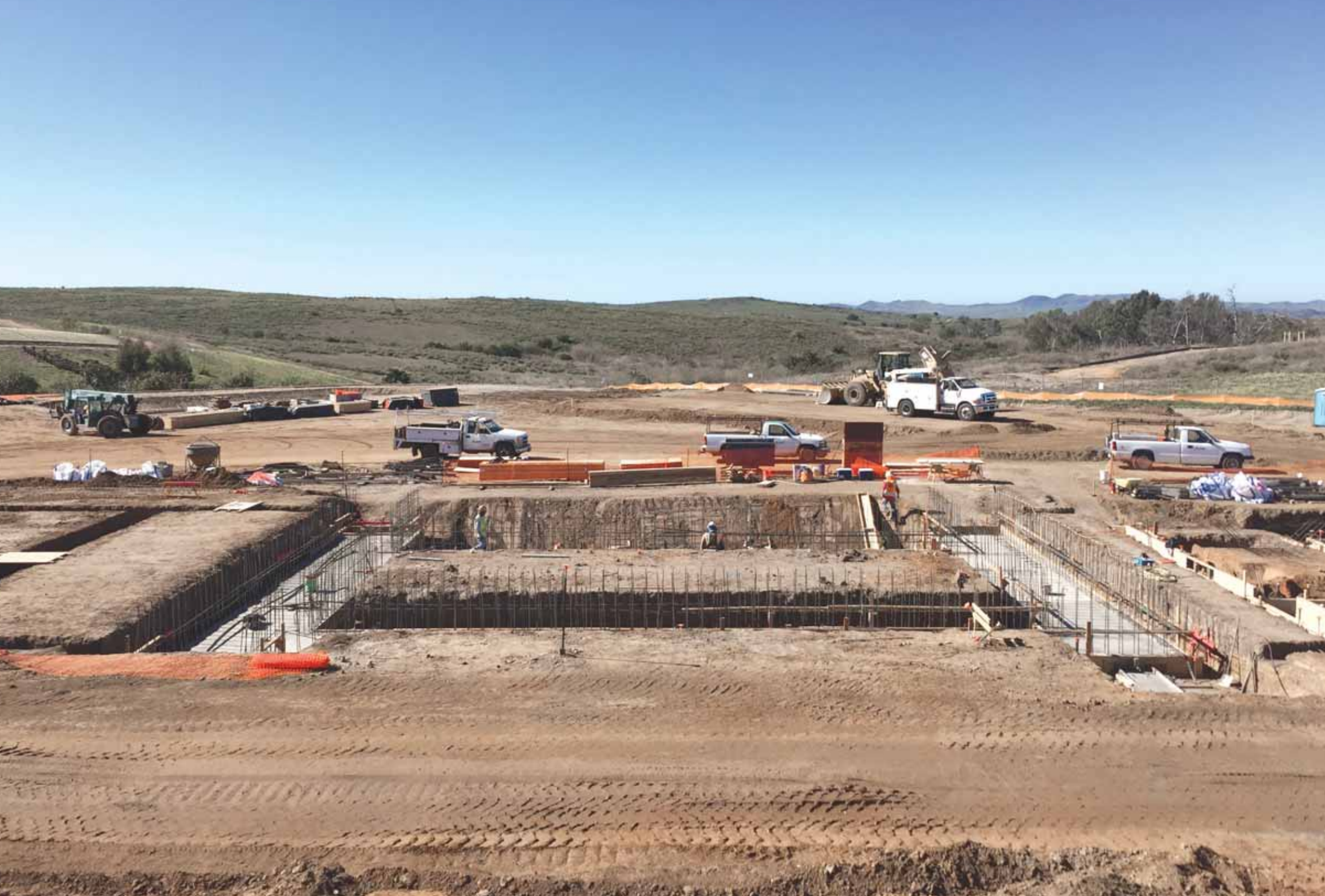
Above: Construction of the water treatment plant on Alturas Road for the Santa Margarita Conjunctive Use Project. Courtesy of FPUD
