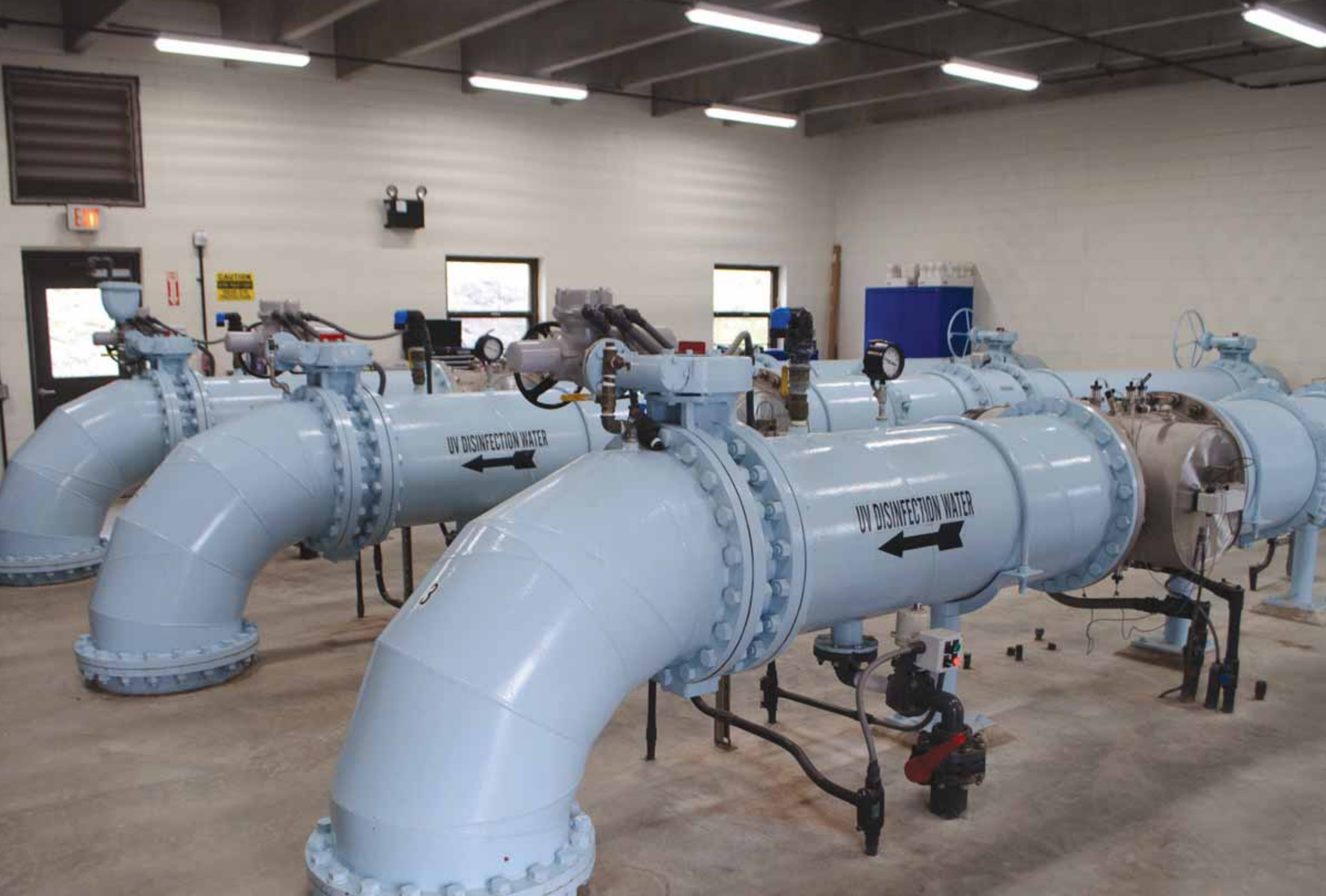
Above: Ultraviolet filtration equipment, a state-of-the-art disinfection process, is in use at the Red Mountain Dam. Courtesy of FPUD
