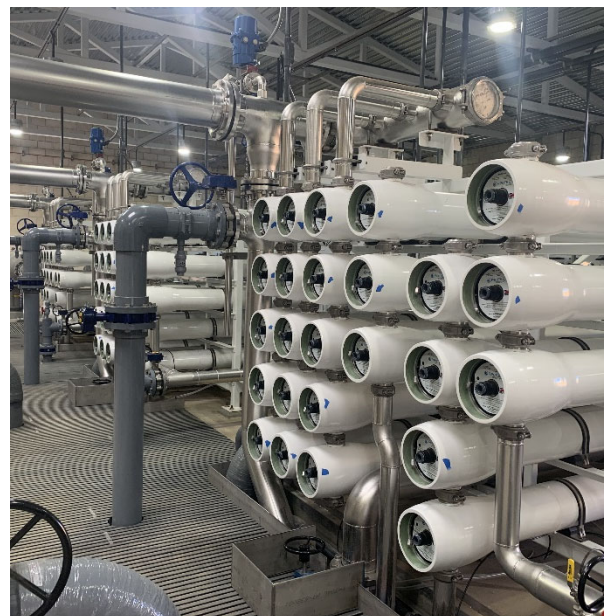
Our state-of-the-art treatment plant has been up and running since November 2021.
