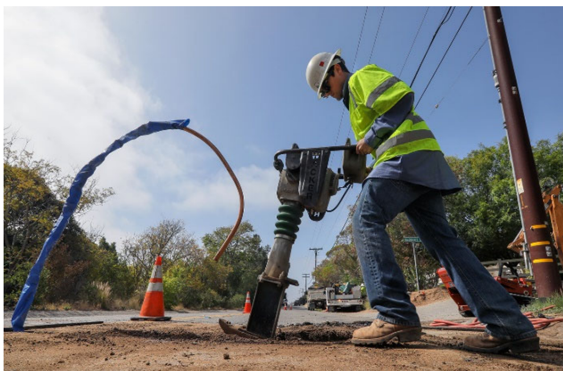
FPUD is working to rehabilitate and replace old pipelines and other aging facilities.
