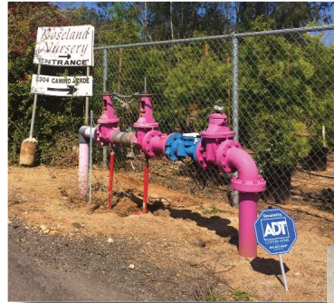
Recycled water program
