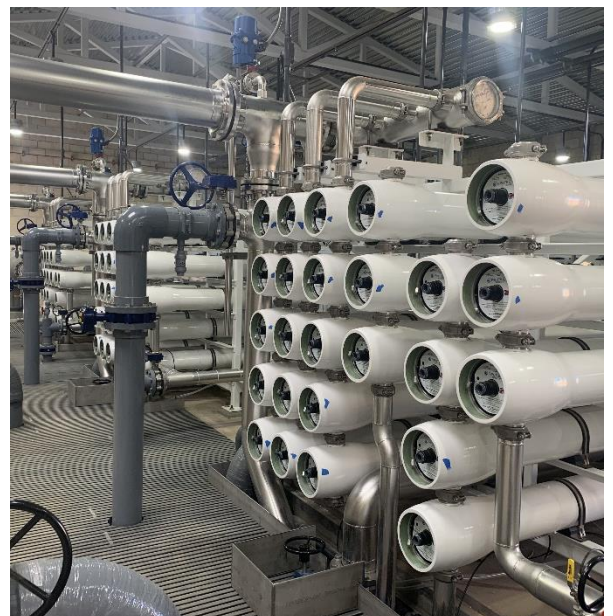
Completion of the Santa Margarita Conjunctive Use Project will reduce reliance on imported water saving customers money. Our state-of-the-art treatment plant has been up and running since November 2021.
