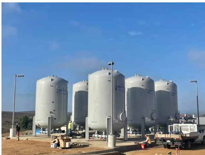
Santa Margarita Groundwater Treatment Plant (SMGTP)
